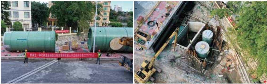
Zhuhai Xiangzhou Axial Flow Pump Station Dual Cylinder Parallel Configuration
