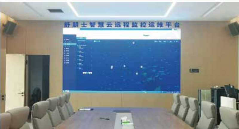
Control Room Remote Monitoring & Operation Platform (control room display)
