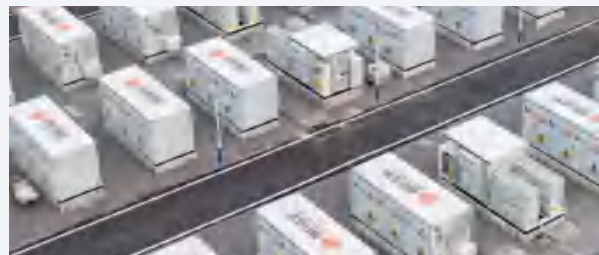
Containerized LFP energy storage station (Liuhe, Jiangsu)
